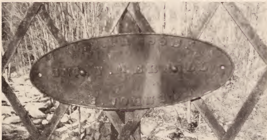
Plaque, north railing, Grist Mill Street Bridge: William S. Pressey, Jno. T. Merrill, Francis B. Johnson.
